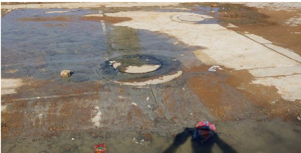
Figure 6: Three images illustrating examples of the presence of the long-term sewage water leaks directly adjacent north and south of the original assessment area which have resulted in confined areas surrounding these leaks, possessing certain anthropogenically induced wetland characteristics
