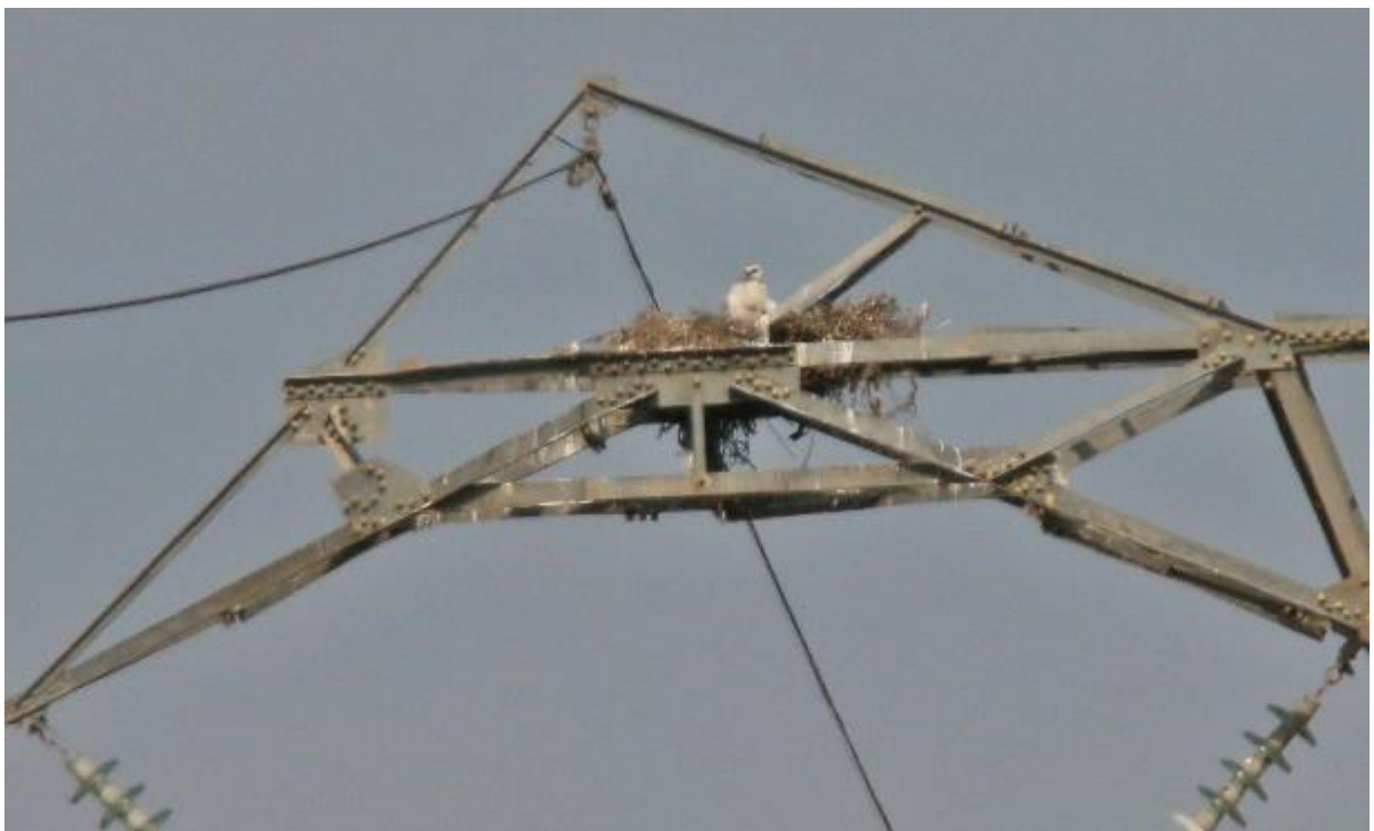
Figure 4: An active Martial Eagle nest on the Aries – Helios 400kV transmission line.
