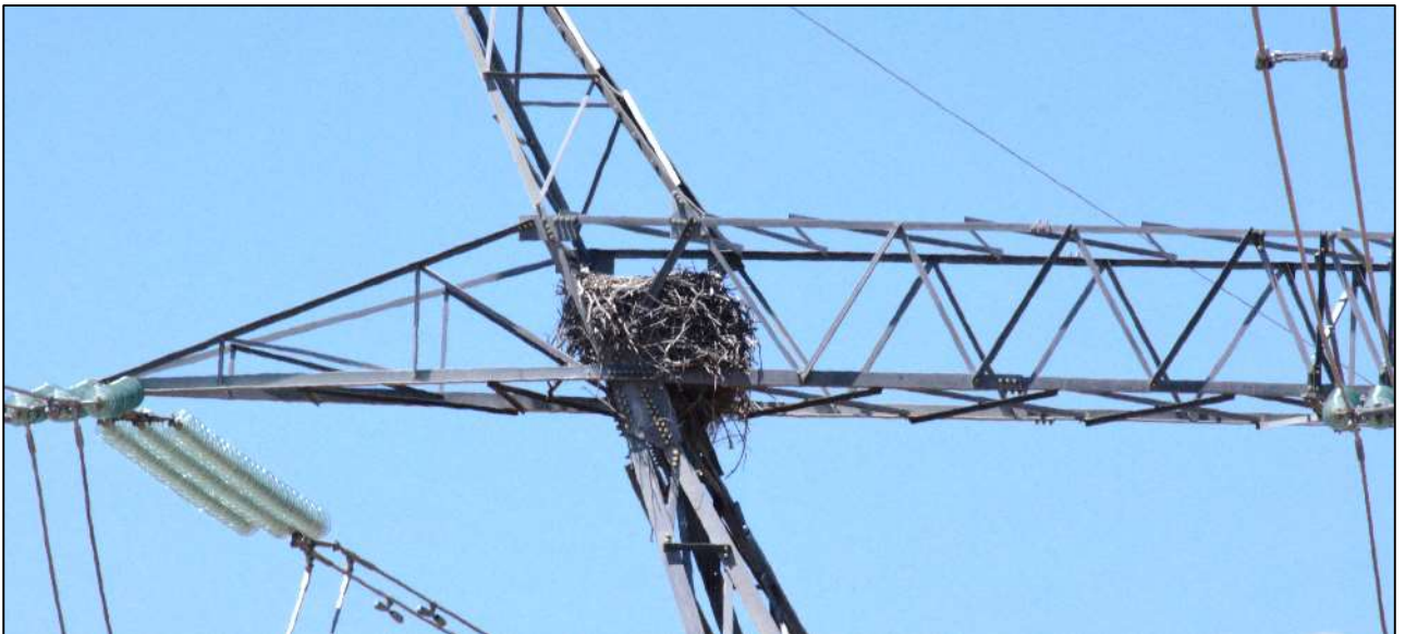
Figure 10: Martial Eagle nest on tower 667 of the Droërvier – Kappa 2 400kV transmission line.
