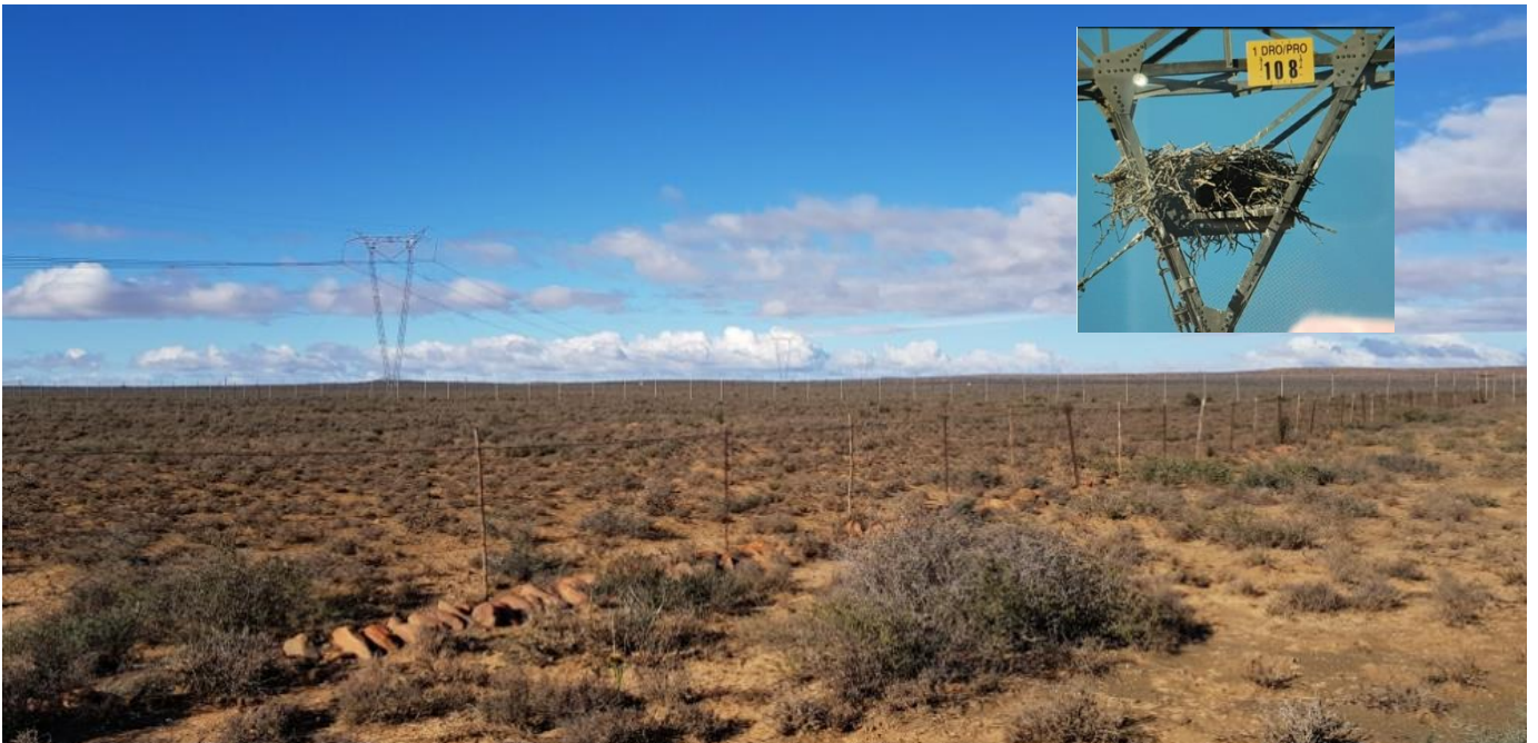
Figure 2: The Droërvier Proteus 400kV HV line that runs approximately 10km west of the study area. The insert shows the Martial Eagle nest on Tower 108.
