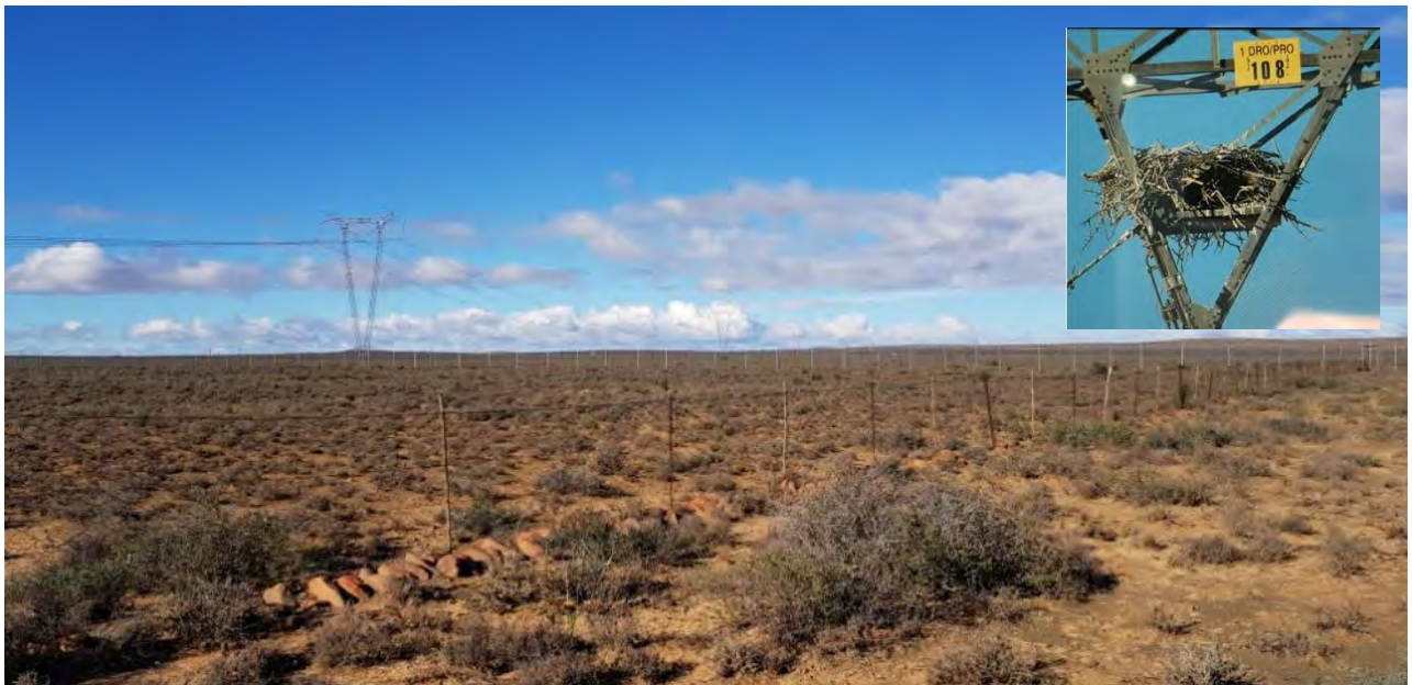
Figure 2: The Droërvier Proteus 400kV HV line that runs through the study area. The insert shows the Martial Eagle nest on Tower 108.
