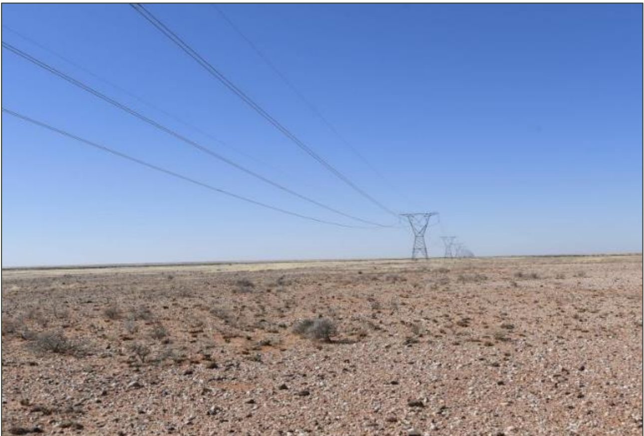
Figure 5: The Aries – Aggeneys 400kV high voltage line that bisects a section of the project site in the south which is used by vultures as a roost in the non-breeding season.
