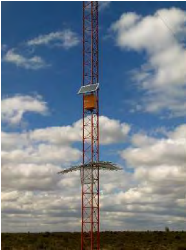
Figure 3: Met mast monitoring system set up
