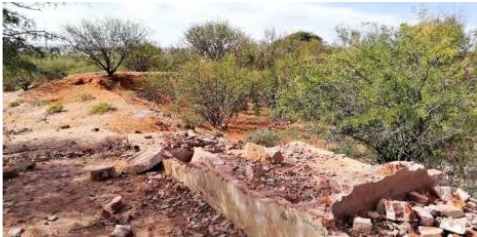
Figure 10 WWTWs Intake structure (Photo Clinton Geysler)
