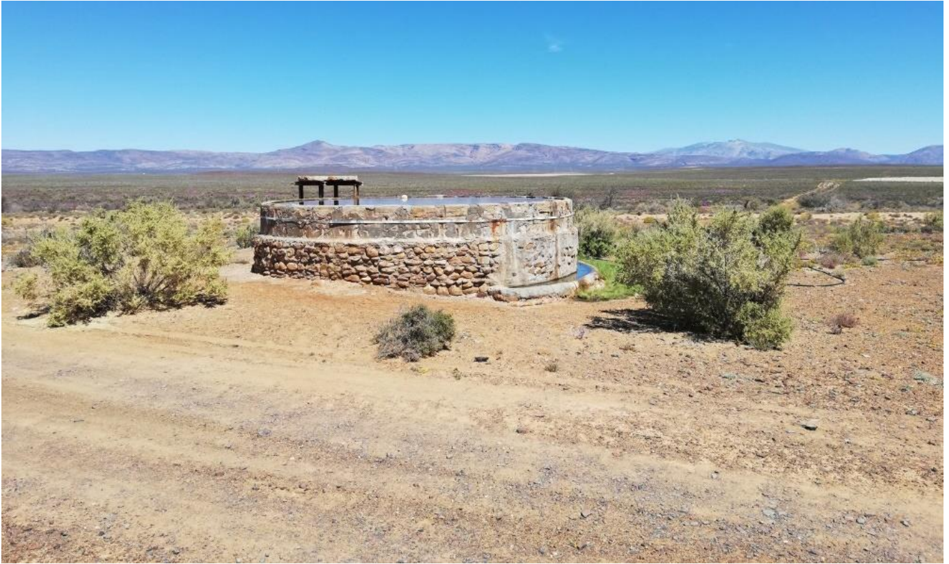
Figure 1: A water reservoir
