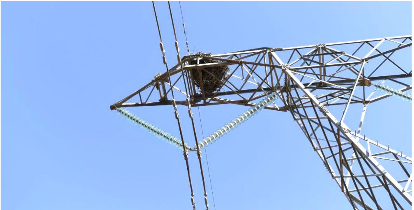
Figure 2: The Kappa Muldersvlei 1 400kV HV line that runs through the PAOI with a Martial Eagle nest on Tower 26.
