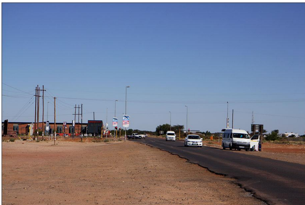
Photo 11: Significant edge break along the R380
