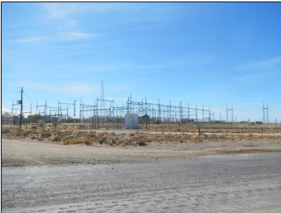
Figure 17: View of Helios Substation
