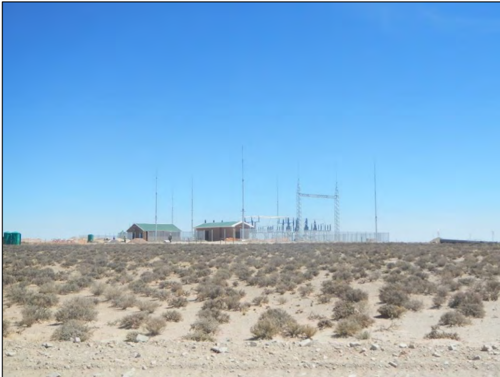
Figure 20: View of the on-site Khobab IPP Substation which had already been constructed during the time of the in-field investigation.
