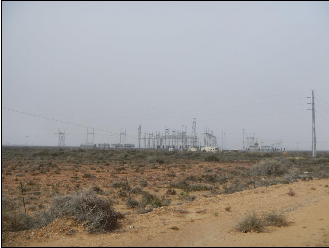
Figure 28: View of the existing Kronos Substation which can be found along the south-western gravel section of the R357 road.
