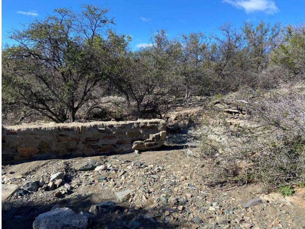
Plate 4: Several small weirs were found within the steeper valleys through-out the study area, most no longer functional
