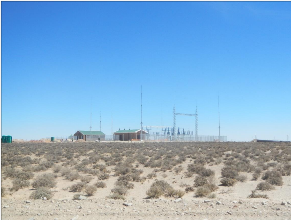
Figure 21: Khobab Wind Farm onsite substation.
