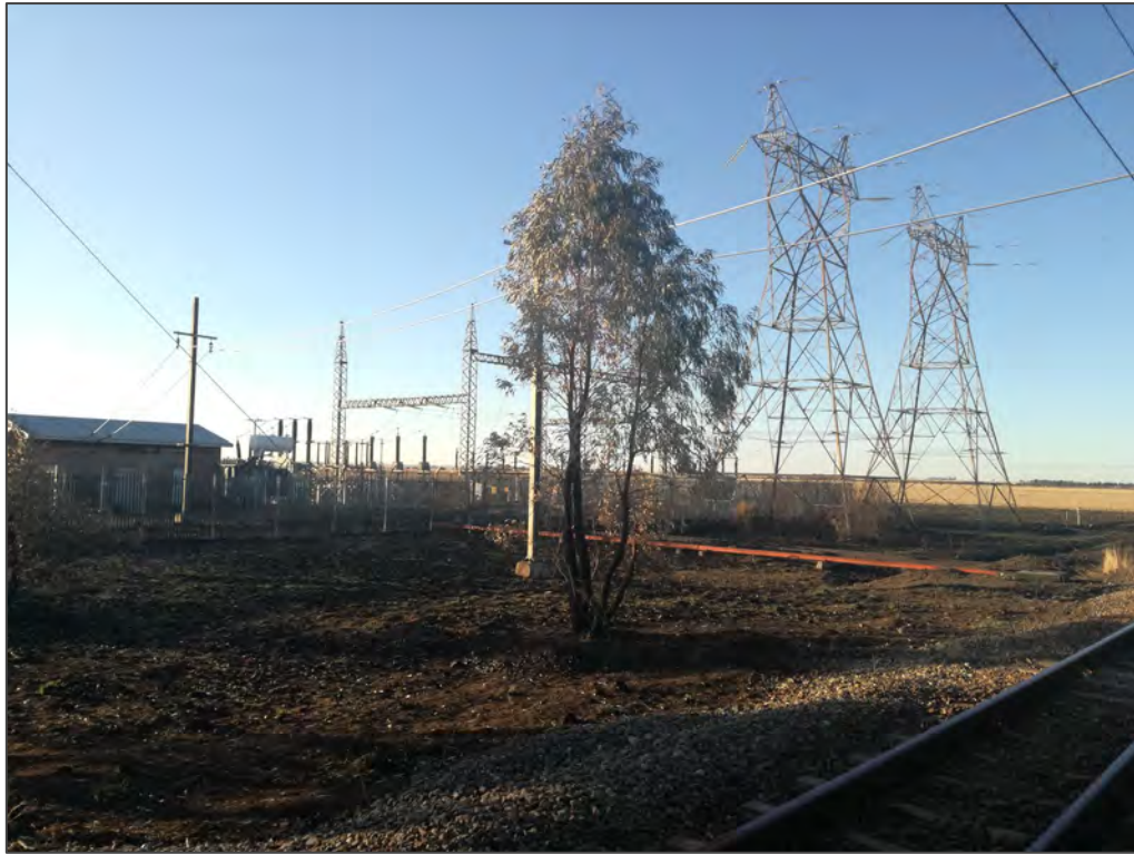
Figure 13: Power lines feeding into the Leeubos TR 132kV Traction Substation
