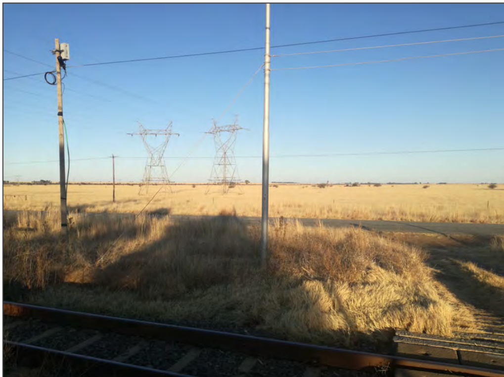
Figure 12: High voltage power lines in the study area
