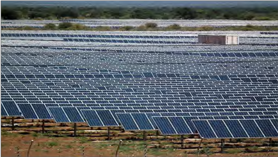
Figure 21: Kathu Solar Power Plant (photo courtesy of “visits to the park”), near Kathu, Northern Cape Province.
