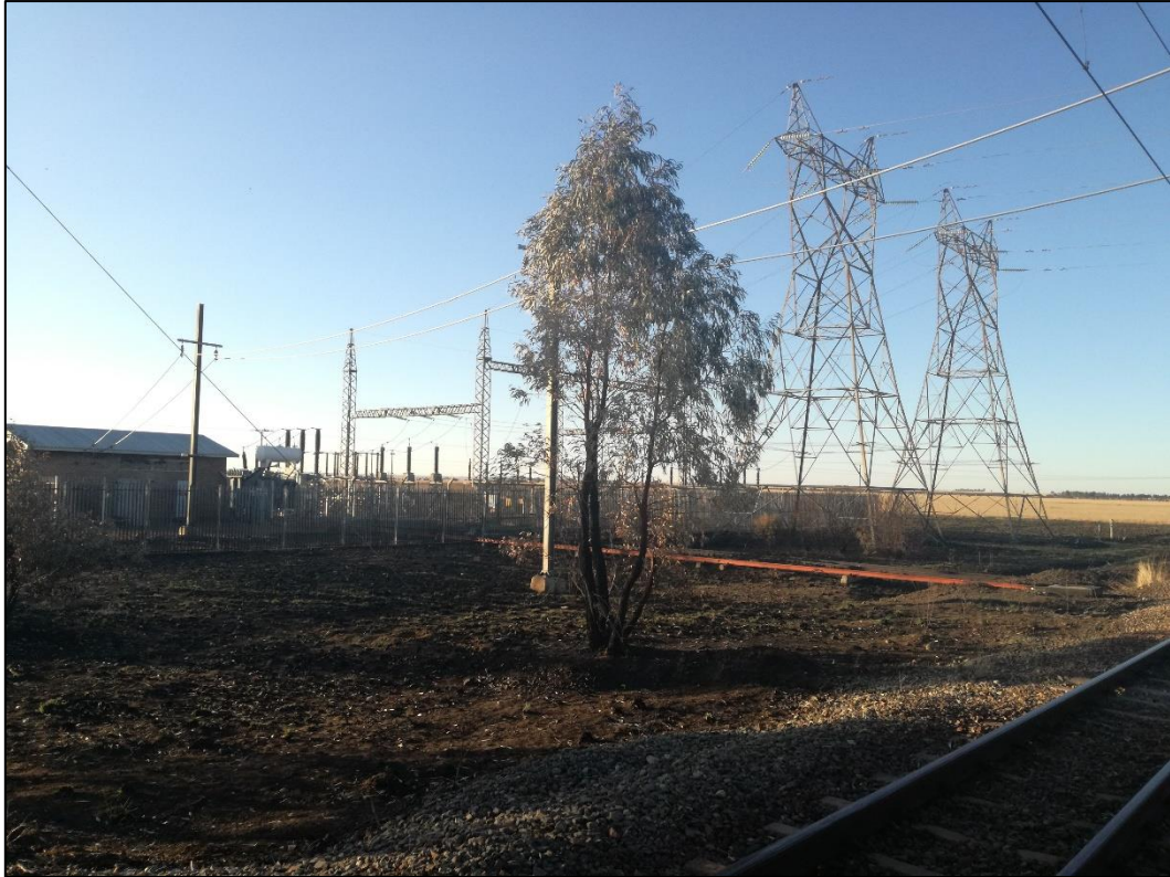
Figure 16: Power lines feeding into the Leeubos TR 132kV Traction Substation
