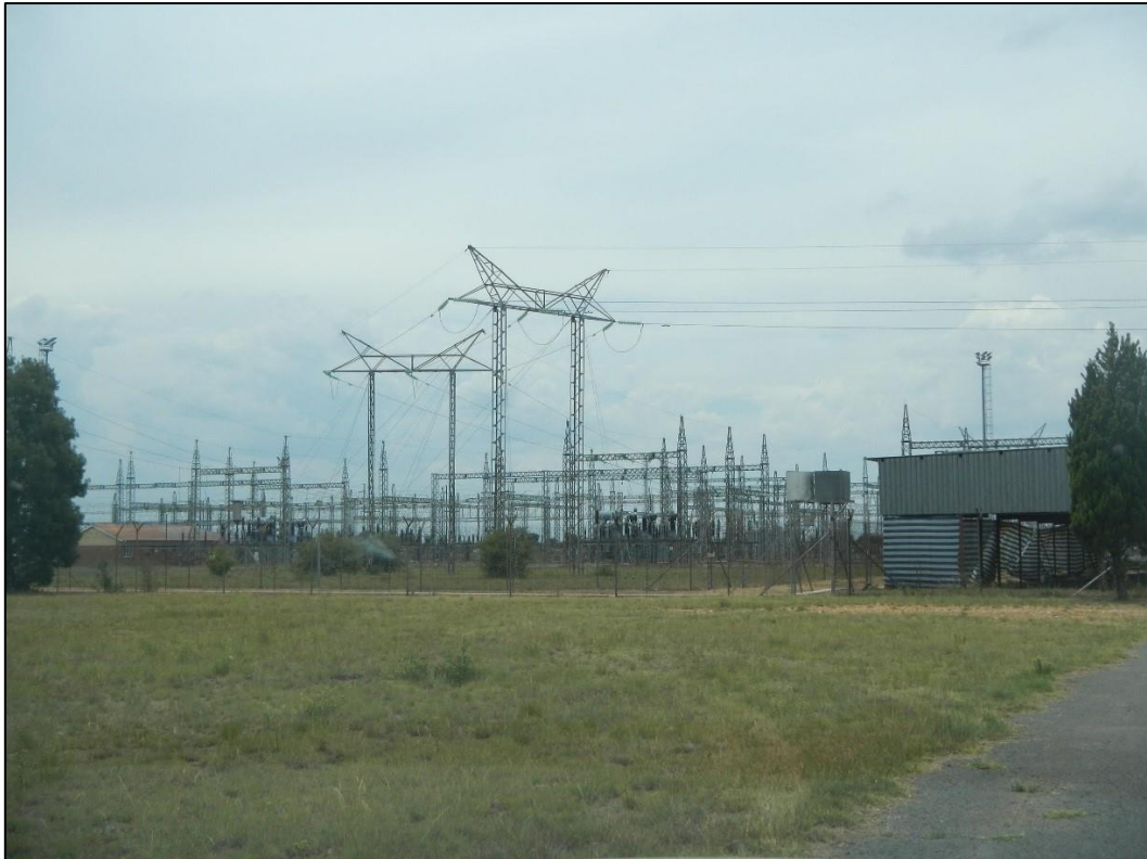
Figure 20: Watershed Substation near Lichtenburg in the North West Province is a good example of a typical Eskom Substation.
