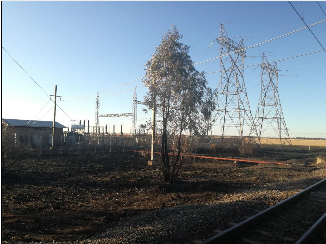
Figure 14: Power lines feeding into the Leeubos TR 132kV Traction Substation
