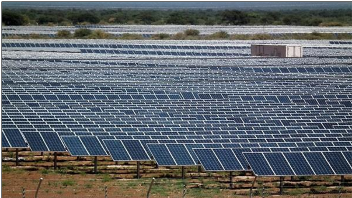
Figure 22: Kathu Solar Power Plant (photo courtesy of “visits to the park”), near Kathu, Northern Cape Province.
