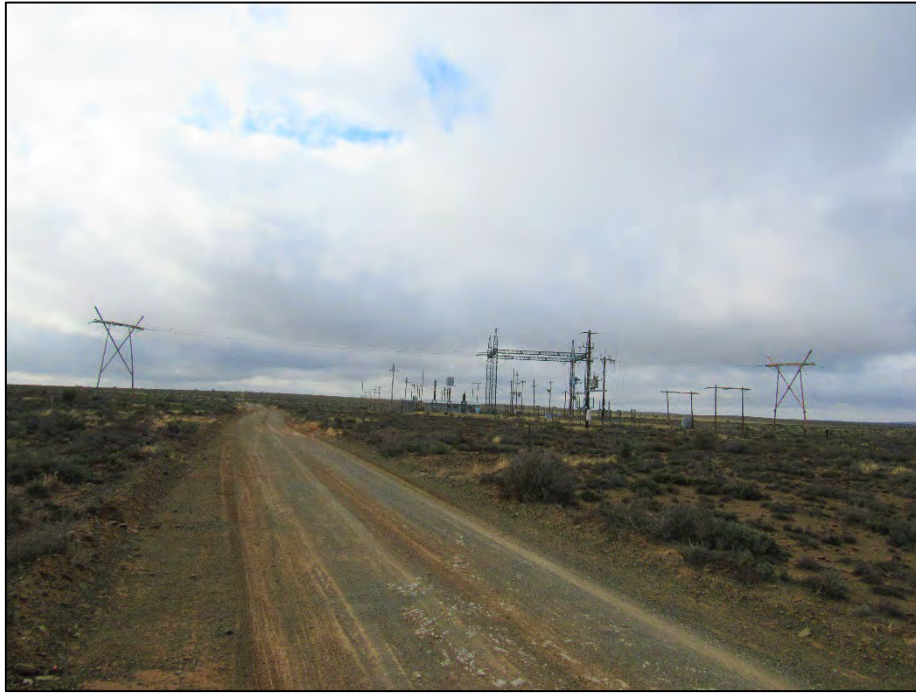
Figure 25: 22kV power lines and associated substation south of the Koup 1 WEF application site, adjacent to the N12.
