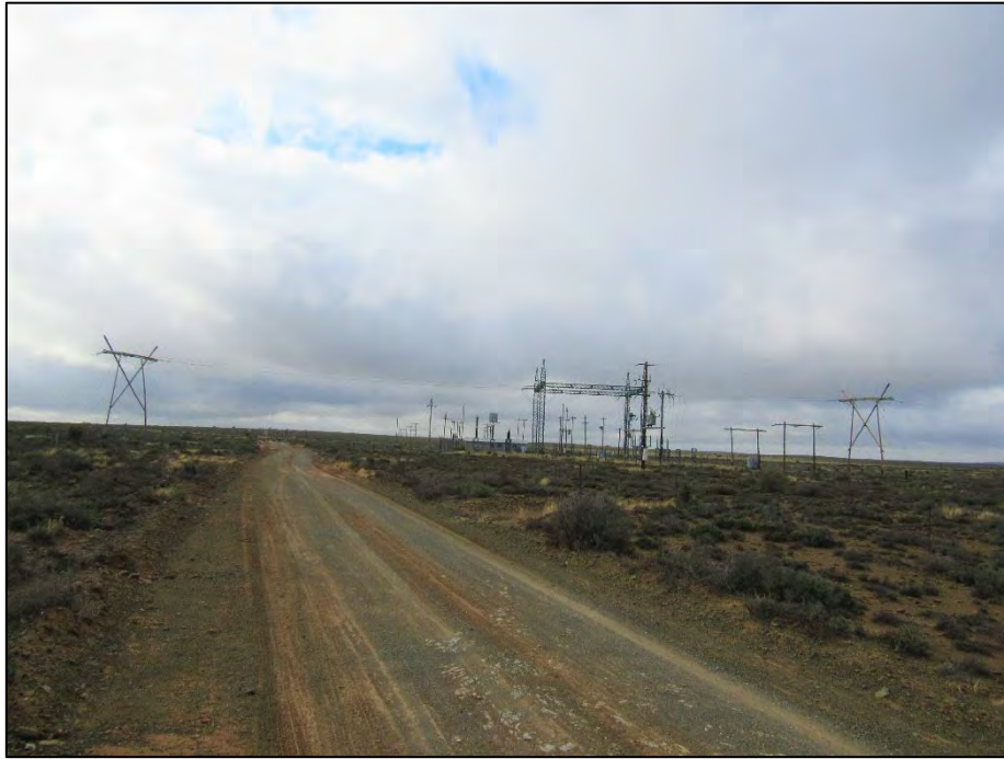
Figure 25: 22kV power lines and associated substation in the south-eastern sector of the Koups 2 WEF application site, adjacent to the N12.
