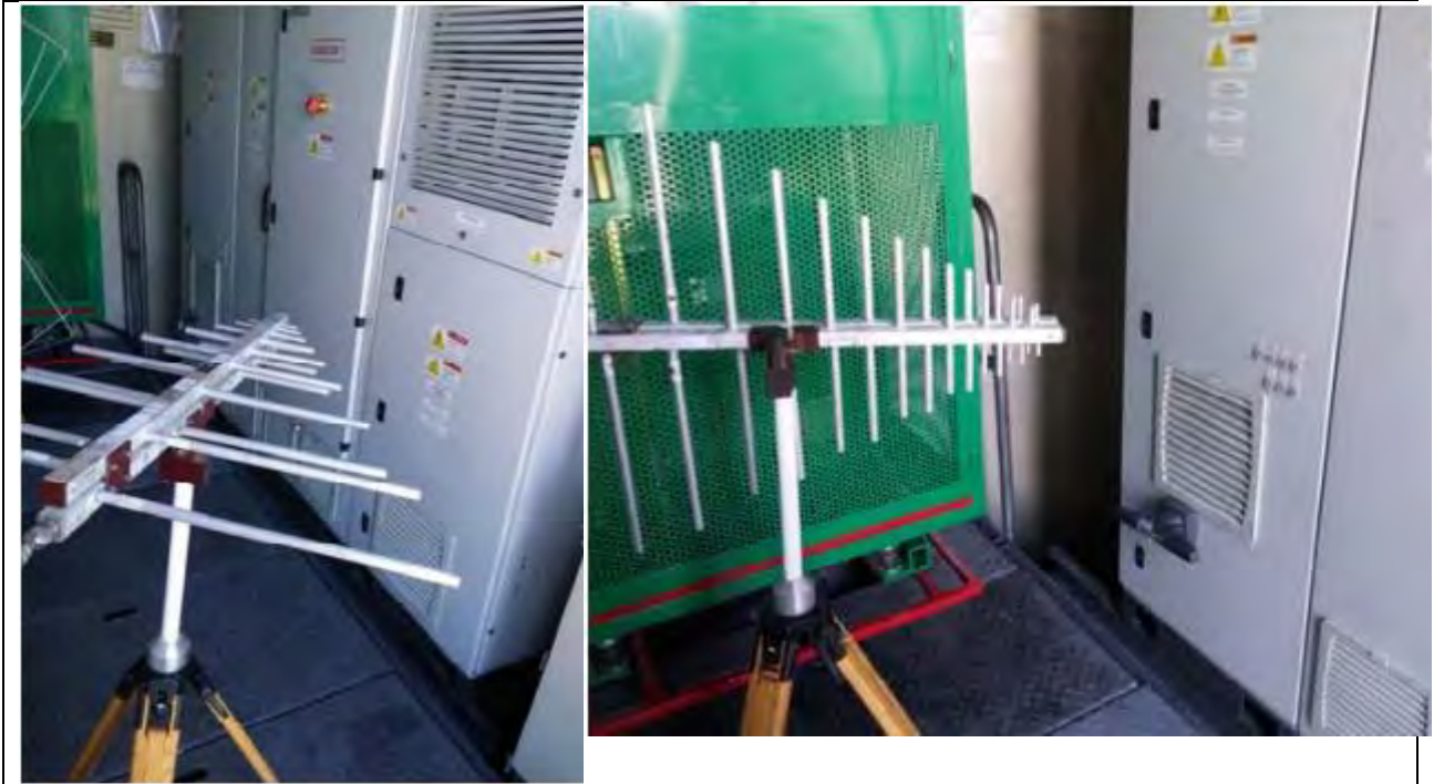
Picture 3: PT0085 Converter cabinet measurements
