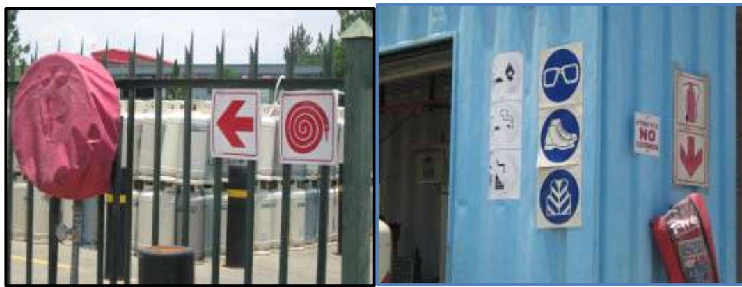
Plate 4: Fire fighting equipment examples and notices
