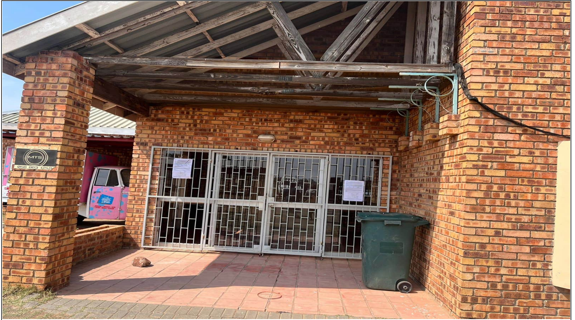
Site notices (Eng & Afr) erected at Dealesville Public Library | 28°39'33.2"S 25°46'18.2"E
