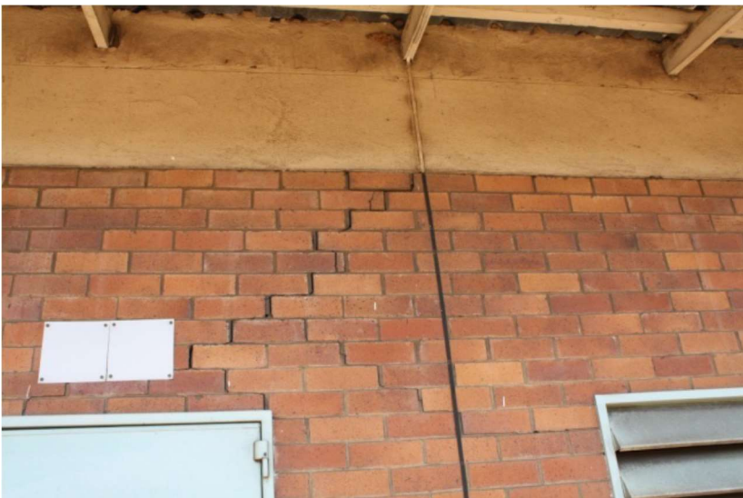
Figure 7: Example of blast induced damage.
