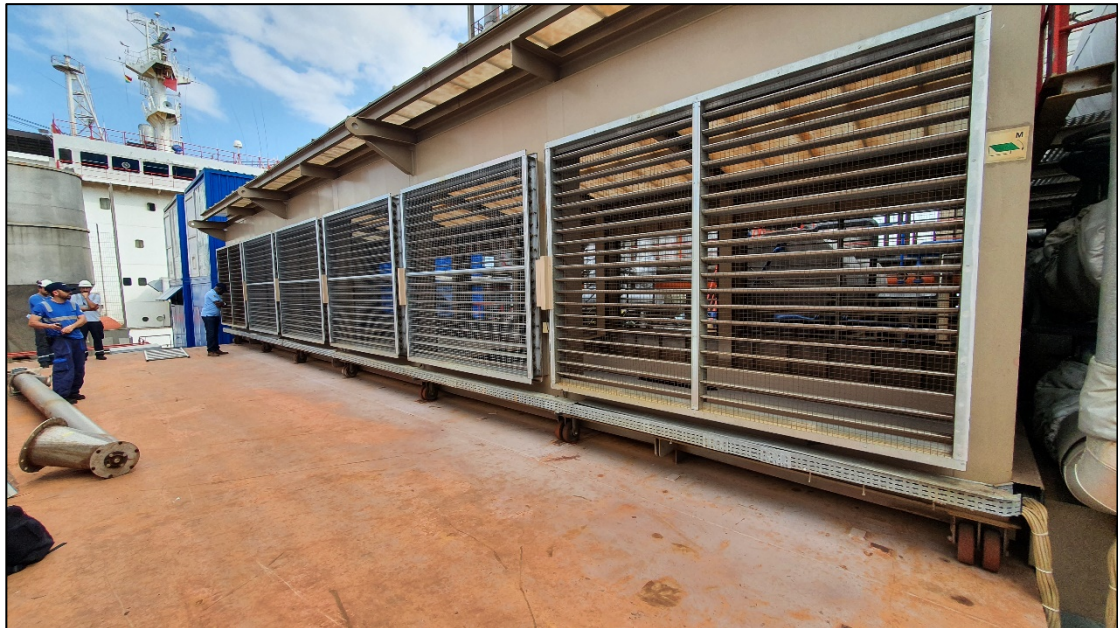
Figure 4: Louvres where Exhaust Heat Outlet is located (Subacoustech, 2022)
