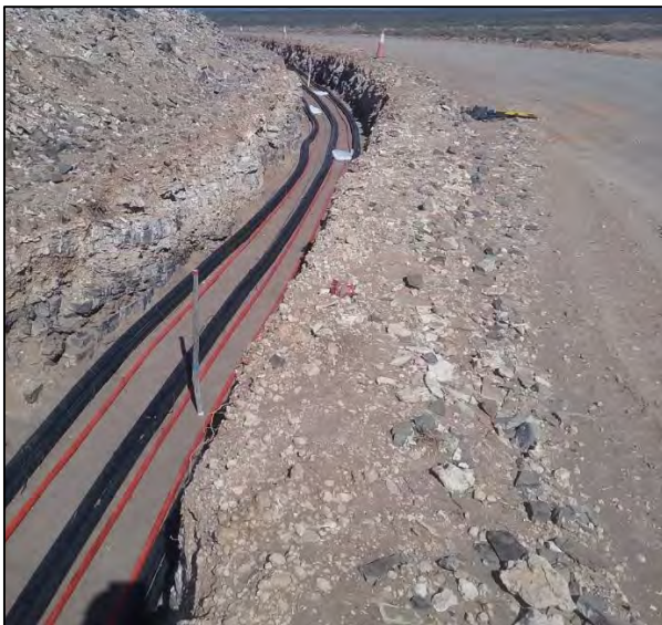
Figure 11.1 - Electrical Connection to Substation along Internal Road
