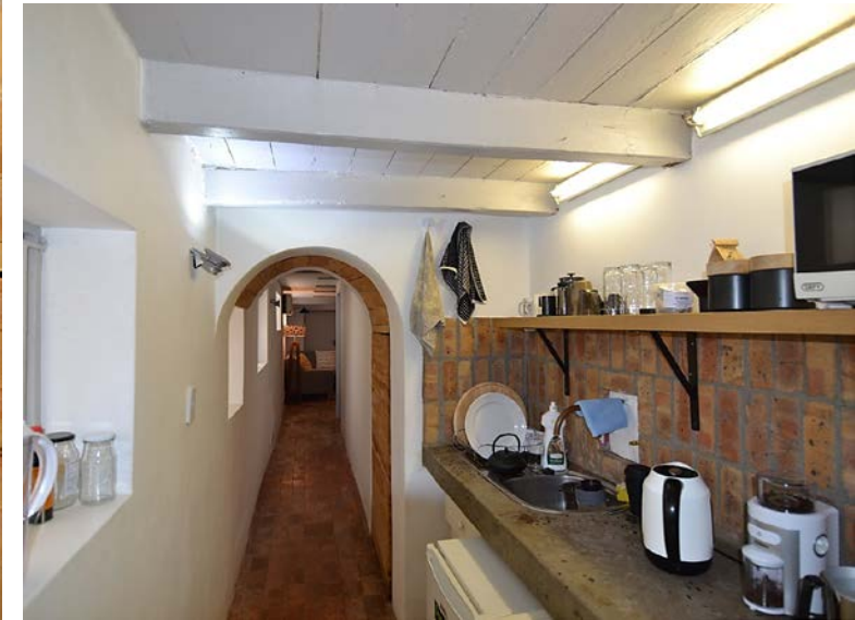
Kitchen and access space. Brick floor, exposed modern painted pine ceiling beams and boards, high level aluminium sliding windows, arch openings(c 1970/80) lined with Poplar and modern kitchen with exposed brickwork splash back wall (2013/14).
