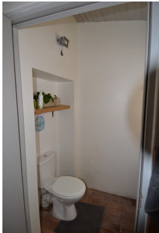
Bathroom spaces. Brick floor, exposed modern painted pine ceiling beams and boards, high level aluminium windows (c 1970/80), modern sanitary ware, exposed modern brickwork splash back and flush new painted doors and frames (c 2013/14).
