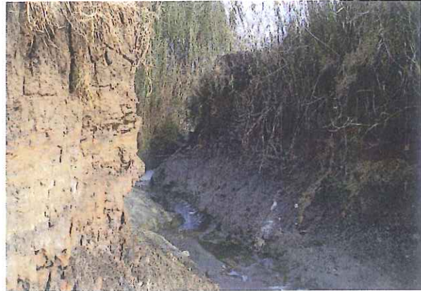
Erosion caused by poor storm water management
