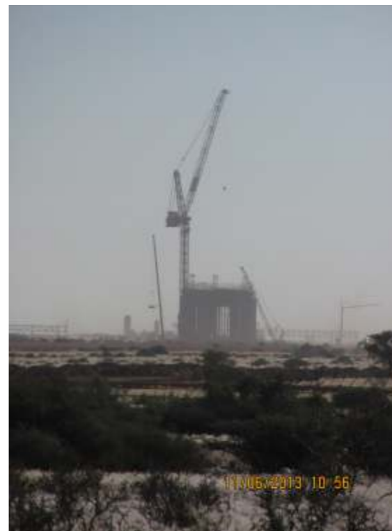
Figure 7: Showing Concentrated Solar Power Plant (CSP) currently under construction on an adjacent property.
