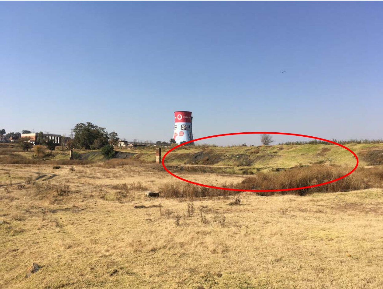
13. Downstream slope. Not maintained, in poor condition and very irregular profiles
