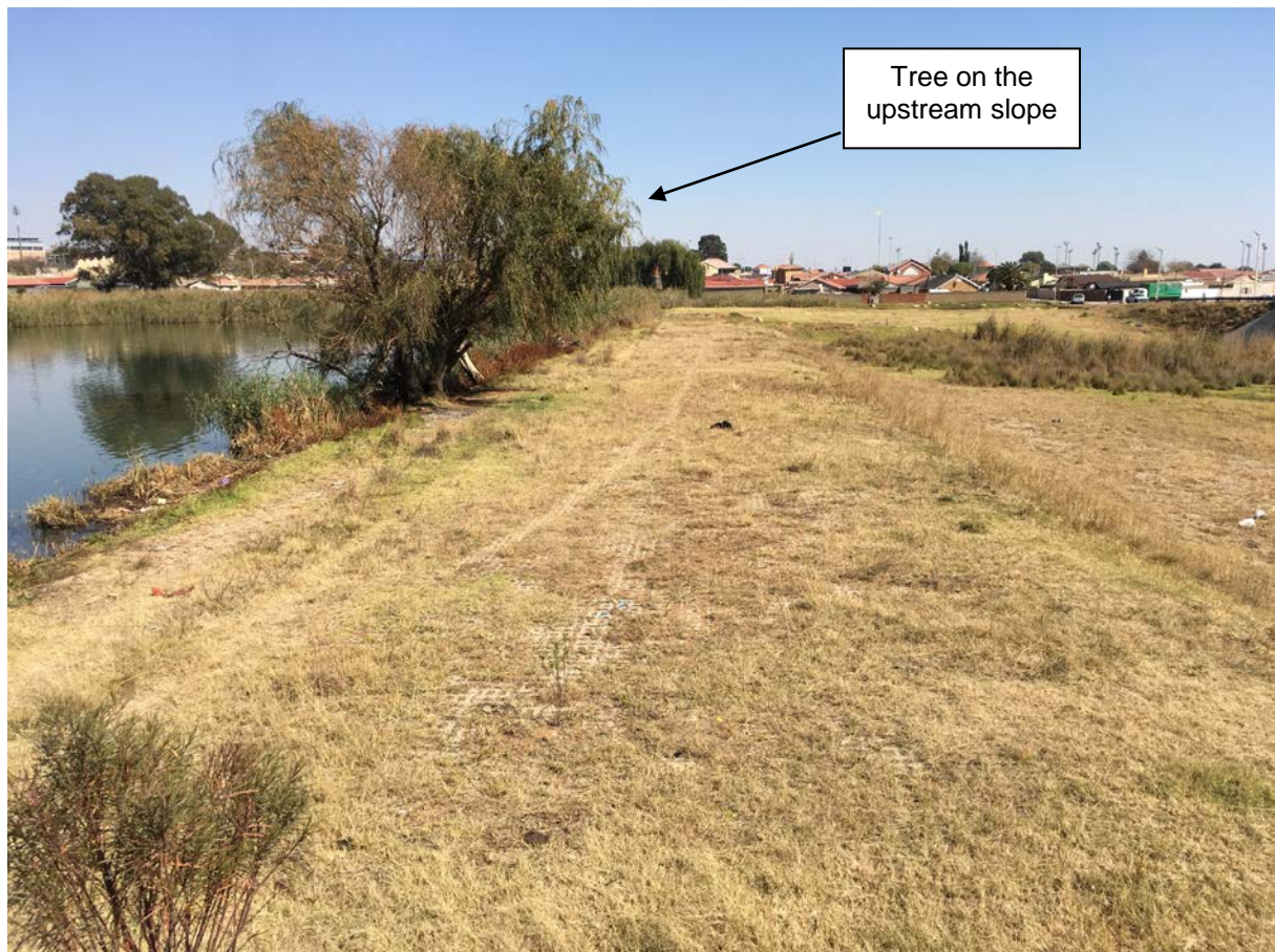
4. View of Auxiliary Spillway showing large tree on the upstream
