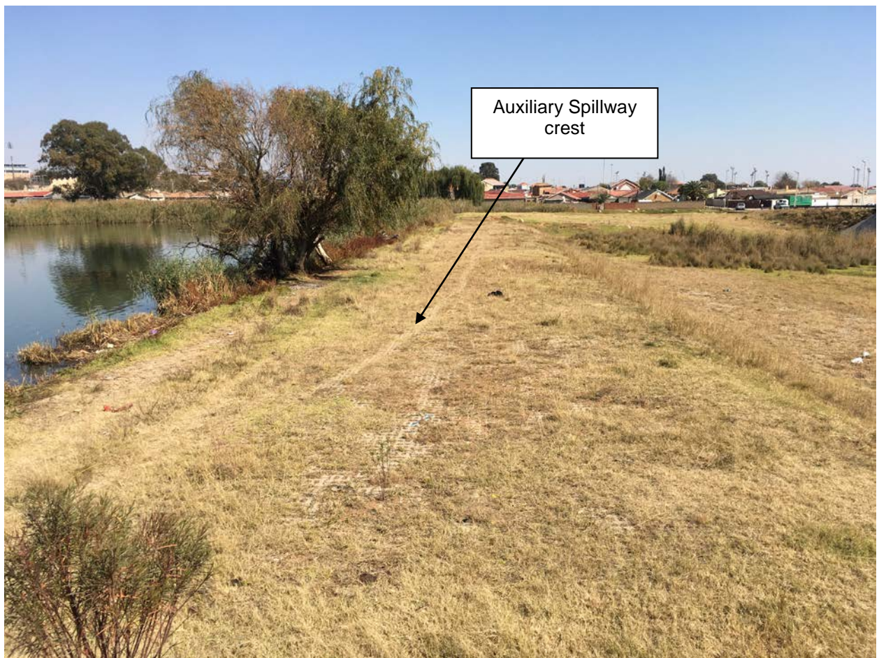
16. Auxiliary Spillway Lack of maintenance, vegetation covering the Armorflex.
