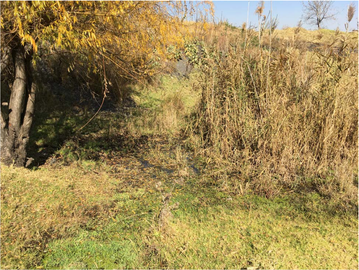
10. Standing water from seepage just downstream of the crest
