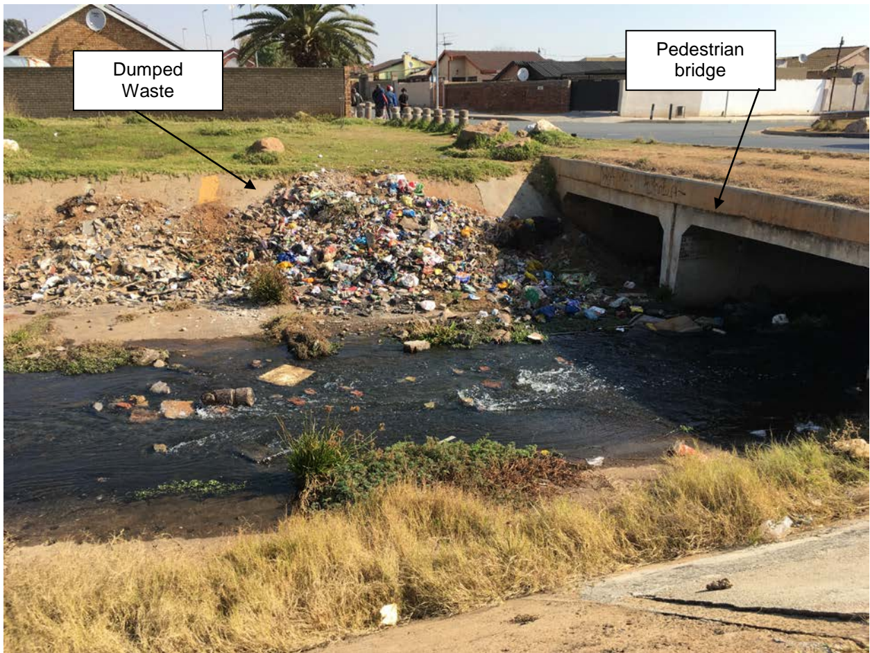
15. Klipspruit Canal and main pedestrian bridge. Used as a dumping spot
