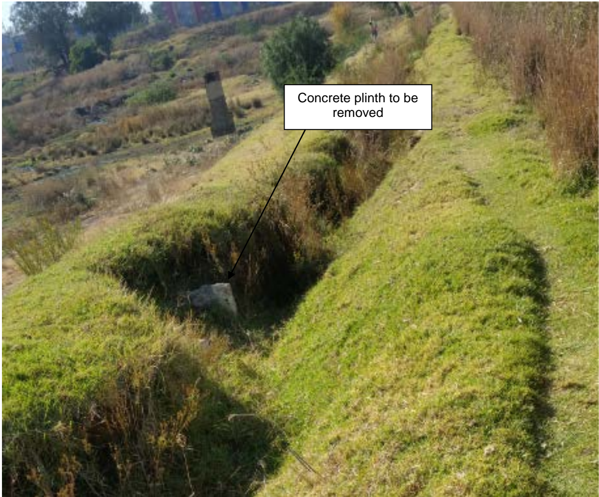
3. Trench on NOC (non-overflow crest) of embankment. Extends for 260 m of 280 m of the crest length, concrete plinth to be removed.
