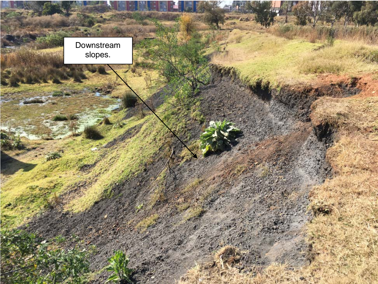
6. General view of downstream slope showing vertical ash dumps (unsafe condition)
