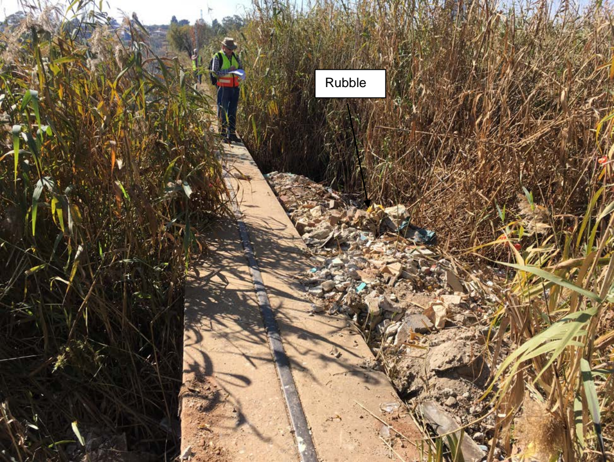
14. Pedestrian bridge across main spillway, Reeds to be removed on both the upstream and downstream side. Rubble to be removed on the upstream side.
