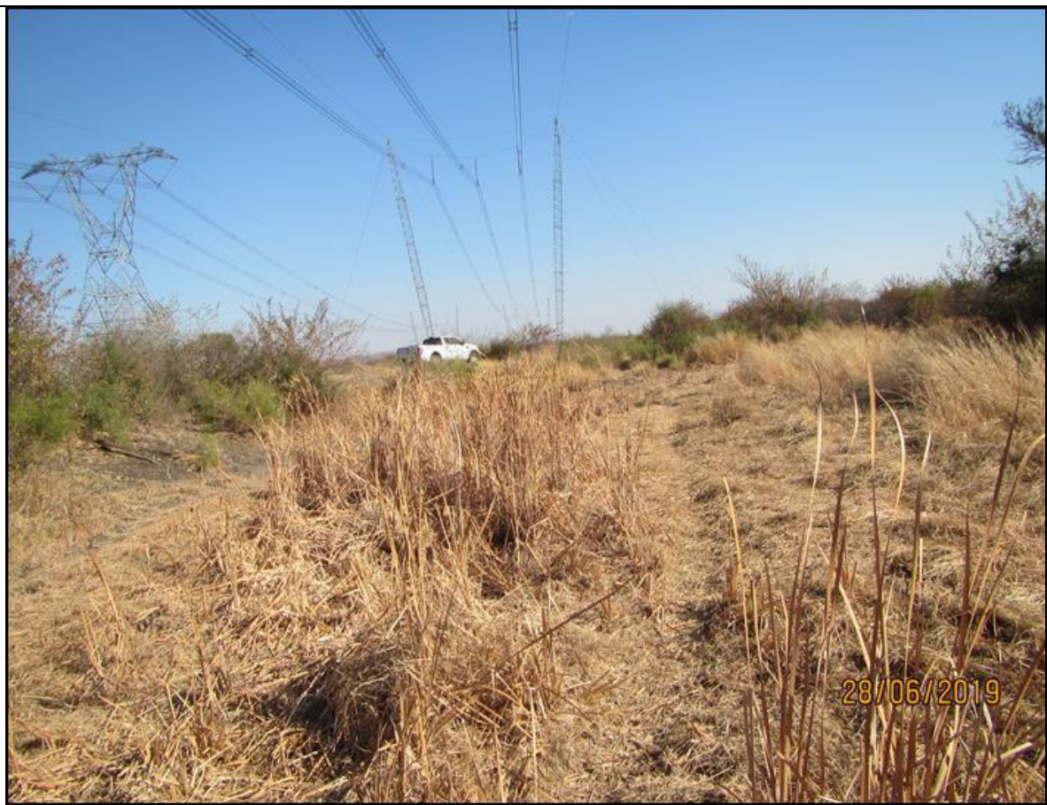
Site 6: Exiting Eskom powerlines within the proposed site location
