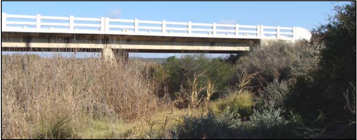
Figure B7: Bridge NB36: View of the bridge from within the watercourse (facing south)
