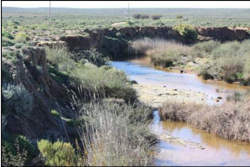
Figure B5: Bridge NB35: View to the upstream of the bridge (facing east)(Photo provided by Aurecon)
