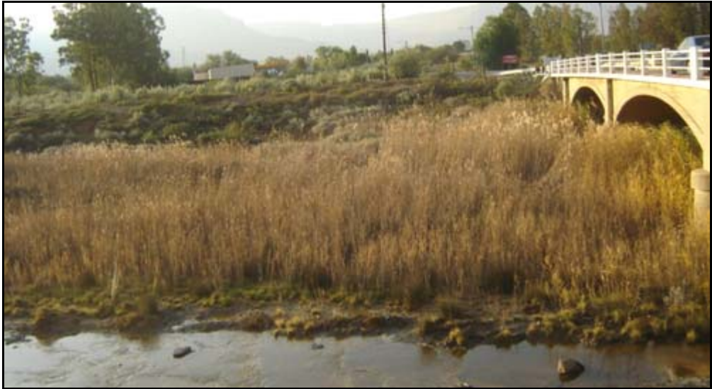
Figure B17: Bridge NB38: View of vegetation in the riverbed downstream of the bridge (facing north-east)
