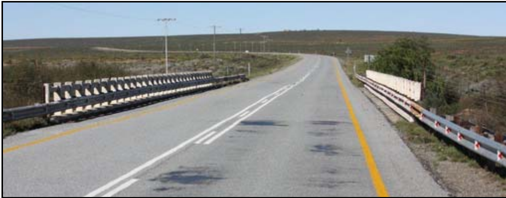
Figure B1: Bridge NB35: View of the R27 across the bridge deck (facing south-east)(Photo provided by Aurecon)
