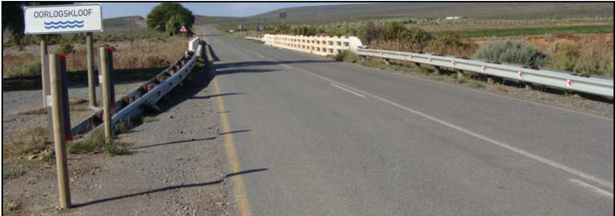
Figure B.6: Bridge NB36: View of the R27 across the bridge deck (facing east)
