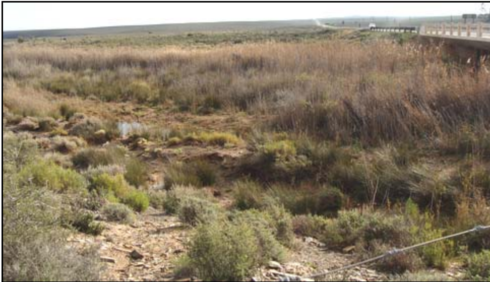
Figure B11: Bridge NB37: View of vegetation in the riverbed downstream of the bridge (facing north-west)
