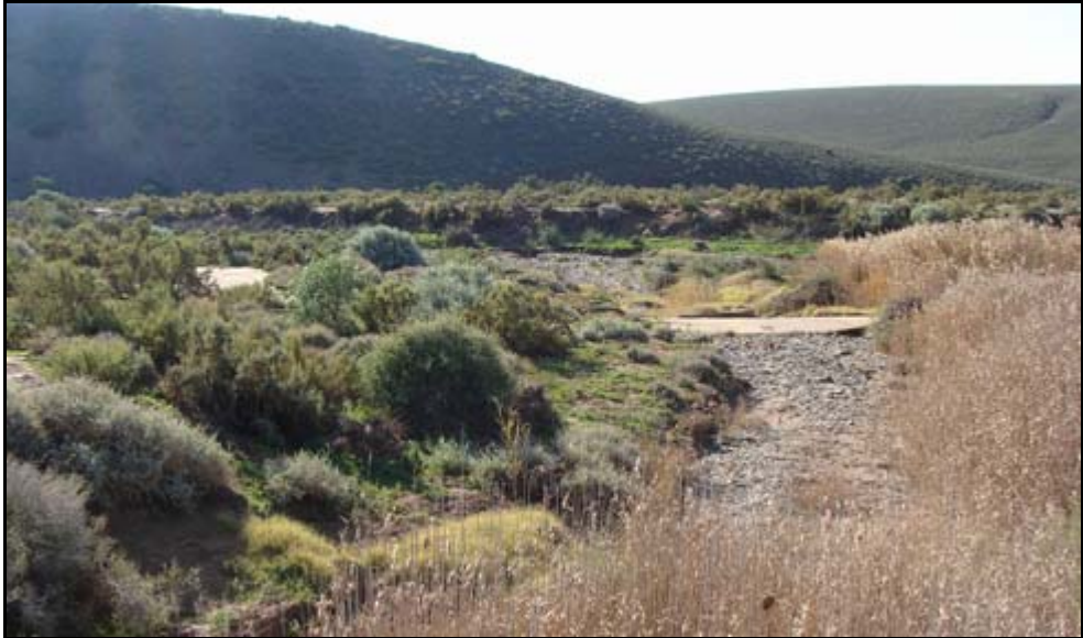
Figure B8: Bridge NB36: View to the downstream of the bridge (facing north-west)
