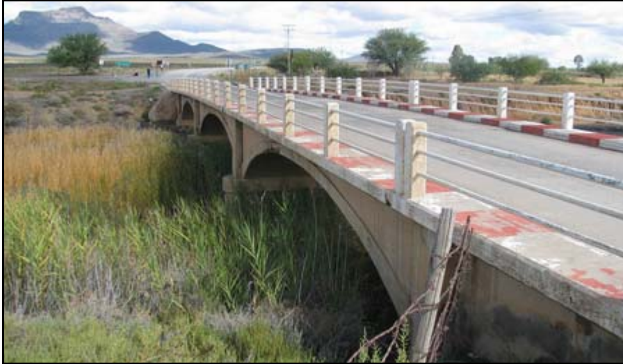
Figure B19: Bridge NB38: View of vegetation in the riverbed upstream of the bridge (facing south-west)(photo provided by T Hart)
