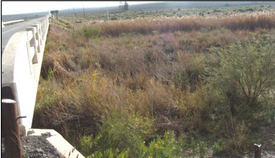
Figure B13: Bridge NB37: View of vegetation in the riverbed upstream of the bridge (facing west)
