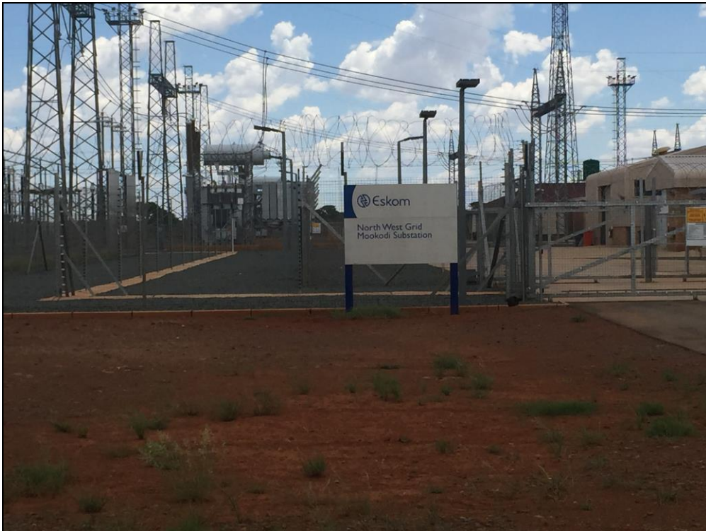
Plate 11: Mookodi Substation (Connection point)
