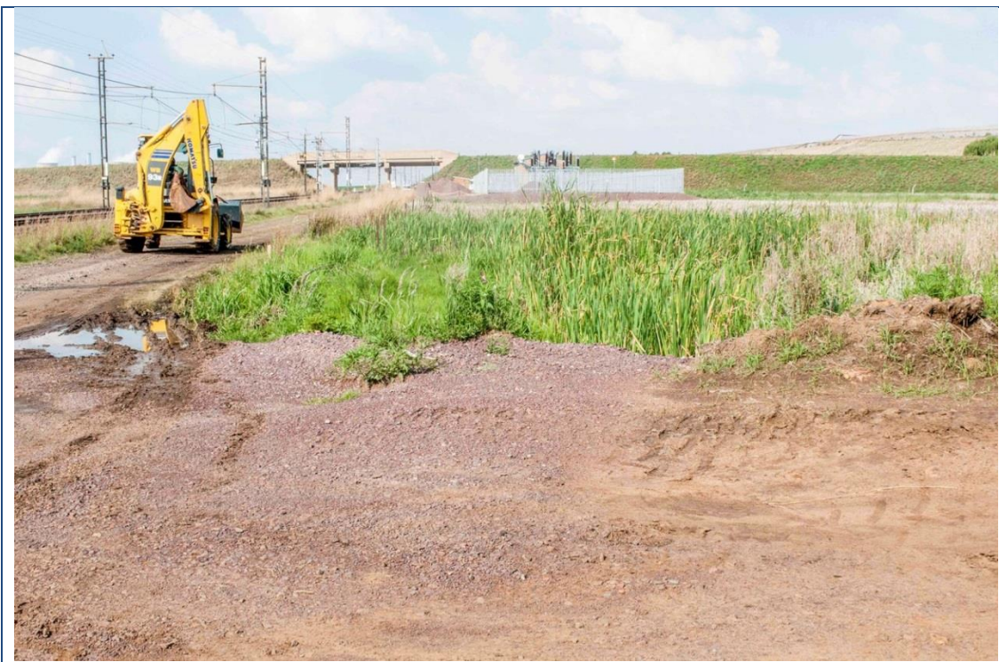
Photo 7: The railway line and service road. Photographed at the site where the new substation is being constructed.
