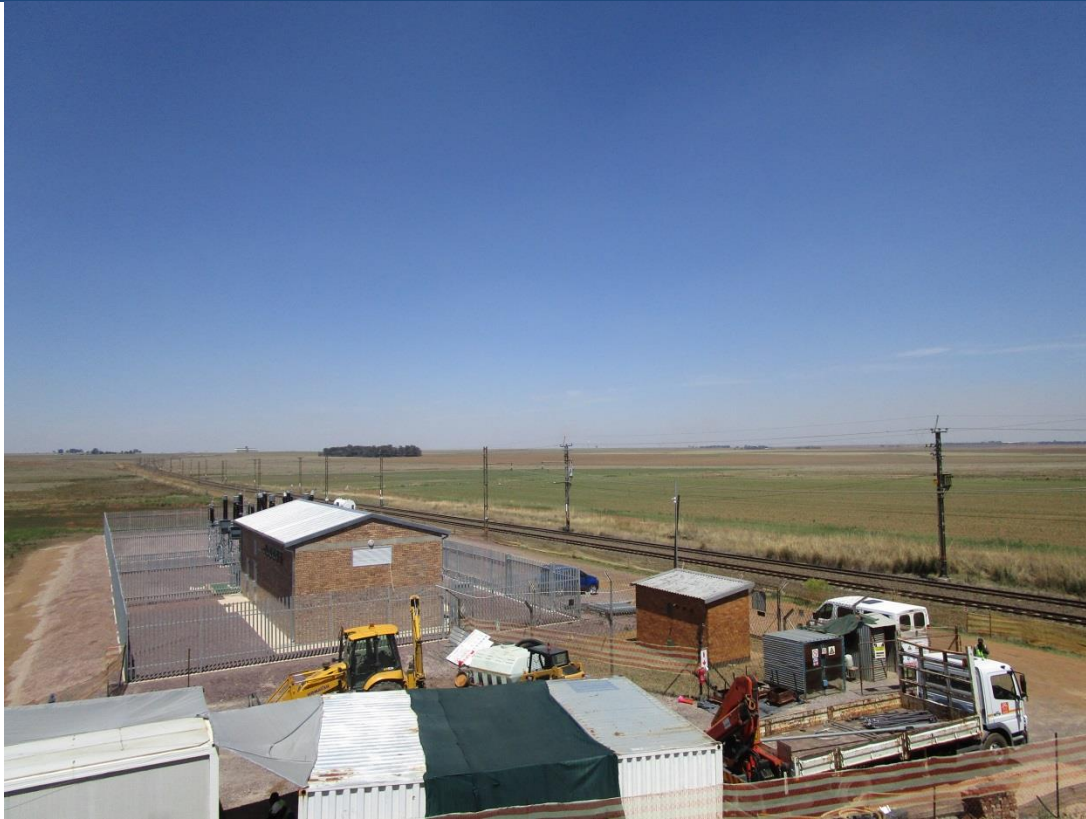
Photo 5: A contractor site camp has been established for the authorised Transnet Boschmanskop traction substation
