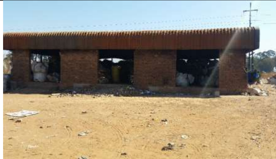
Figure 10: A degraded buy back centre is observed on the western boundary of the site
