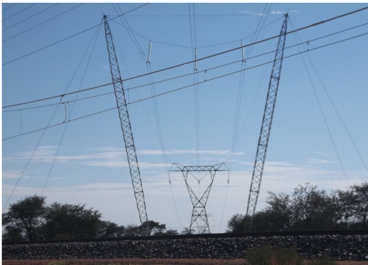
Plate 4: View towards the north west . Photo was taken at the point where the existing 275 kV power line was lifted to make way for the construction of the new Postmasburg – Hotazel railway line.
