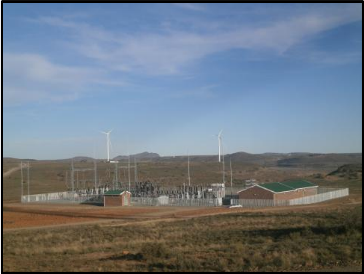
Image of the existing Noblesfontein substation.
