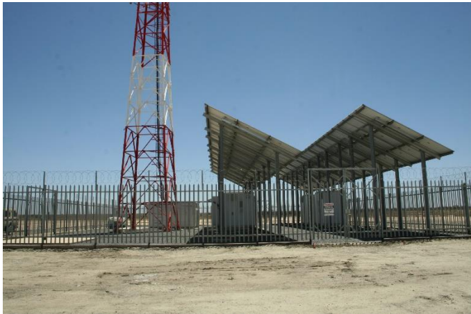
Photo 7: The existing MTN telecommunications mast, and general location of the proposed technical camp. Taken at Point 6
