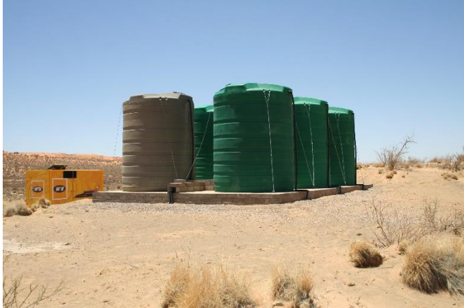
Photo 9: Water storage tanks at the Speedweek camp
