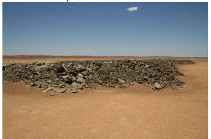
Photo 6: The material is removed by hand and by machinery and consolidated in stockpiles on Hakskeen Pan. Taken at Point 5
