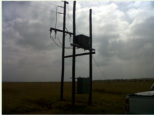
Figure 5 | ESKOM transformer ESKOM has installed a transformer at the site. Electricity will be supplied by ESKOM
