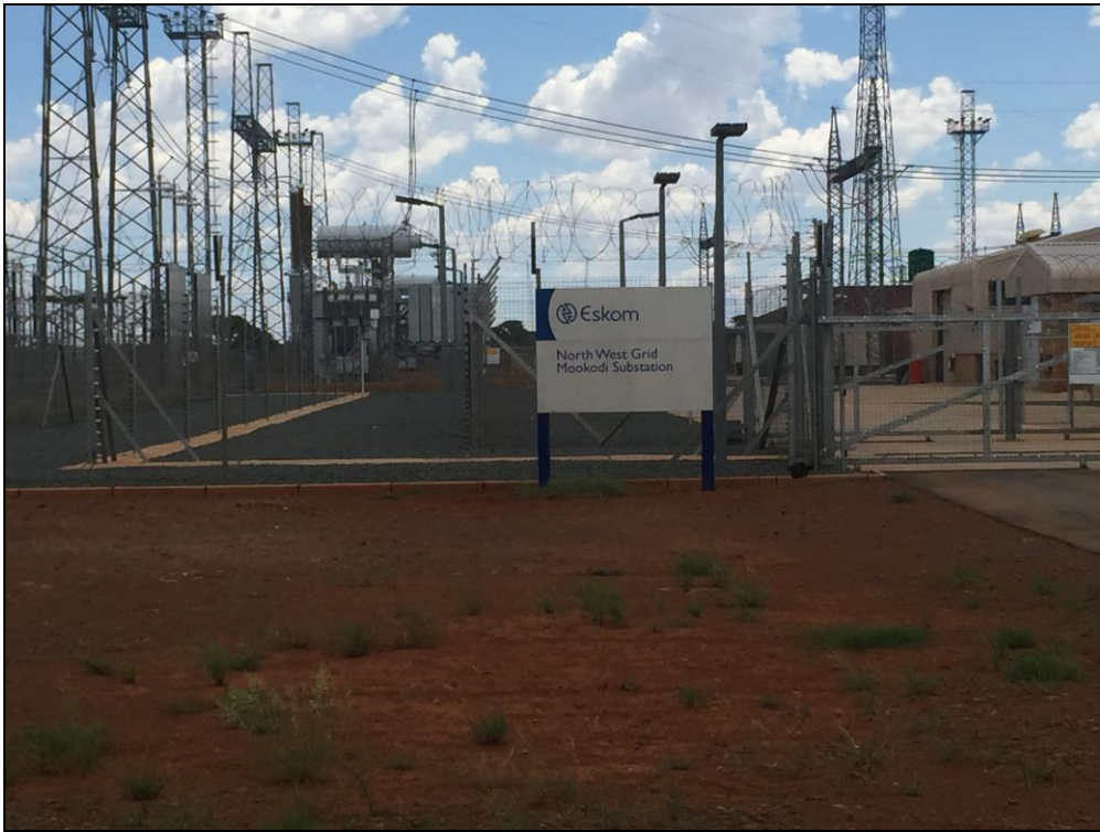
Plate 11: Mookodi Substation (Connection point for Waterloo Solar Park)
