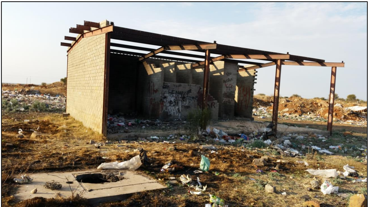
Figure 12: Close up view of the dilapidated structure on site
