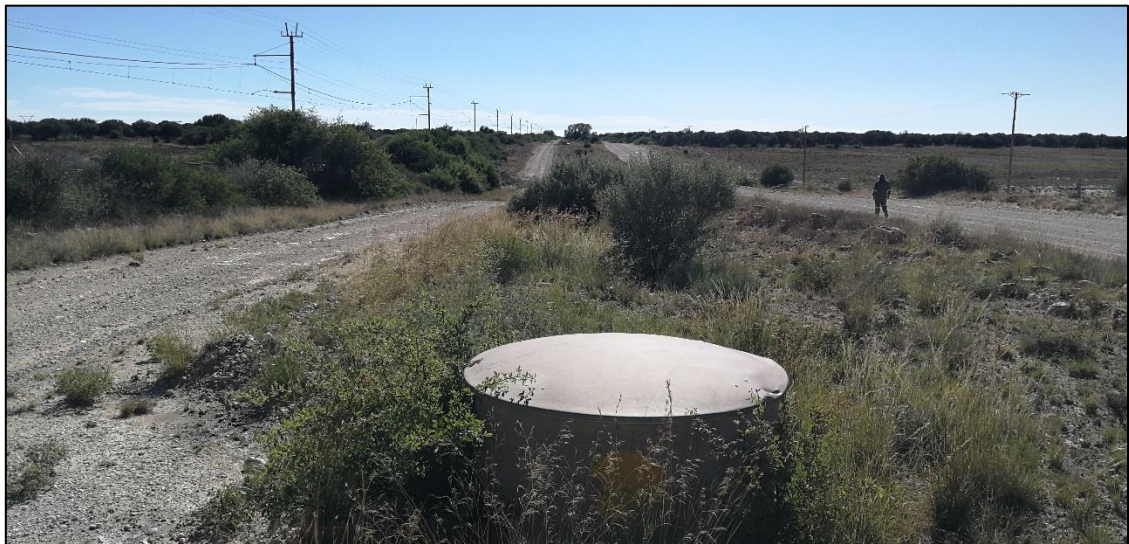
Figure 8: Views along pipeline from Trewill Pump Station to R385 near Lime Acres
