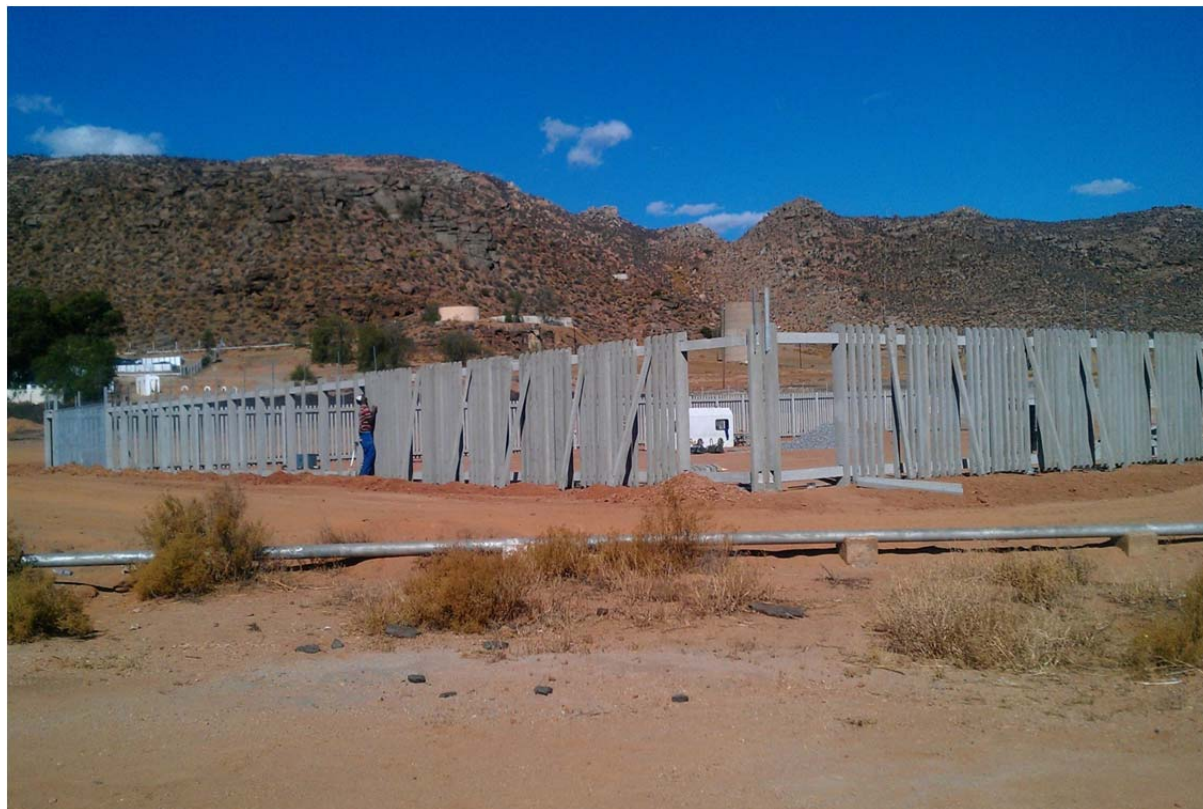
Figure 10: Construction progress at the Nama Koi Substation as seen on the 25 th of January 2012 (this is a Nama Koi Local municipality project)
