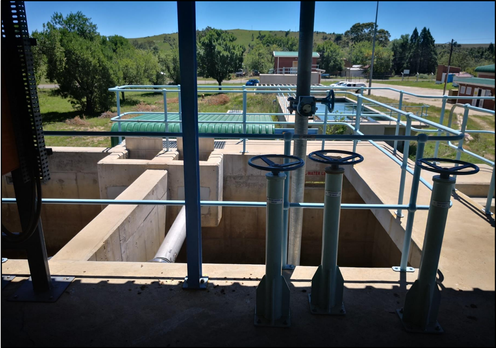
Photo: 1 Lindley Treatment Plant
