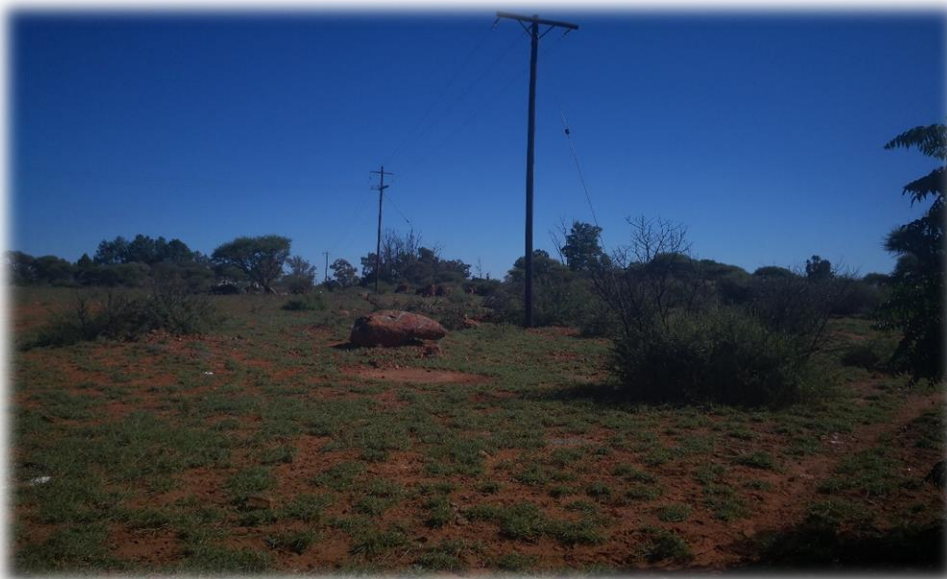
Photo 4: View of the overhead powerline
