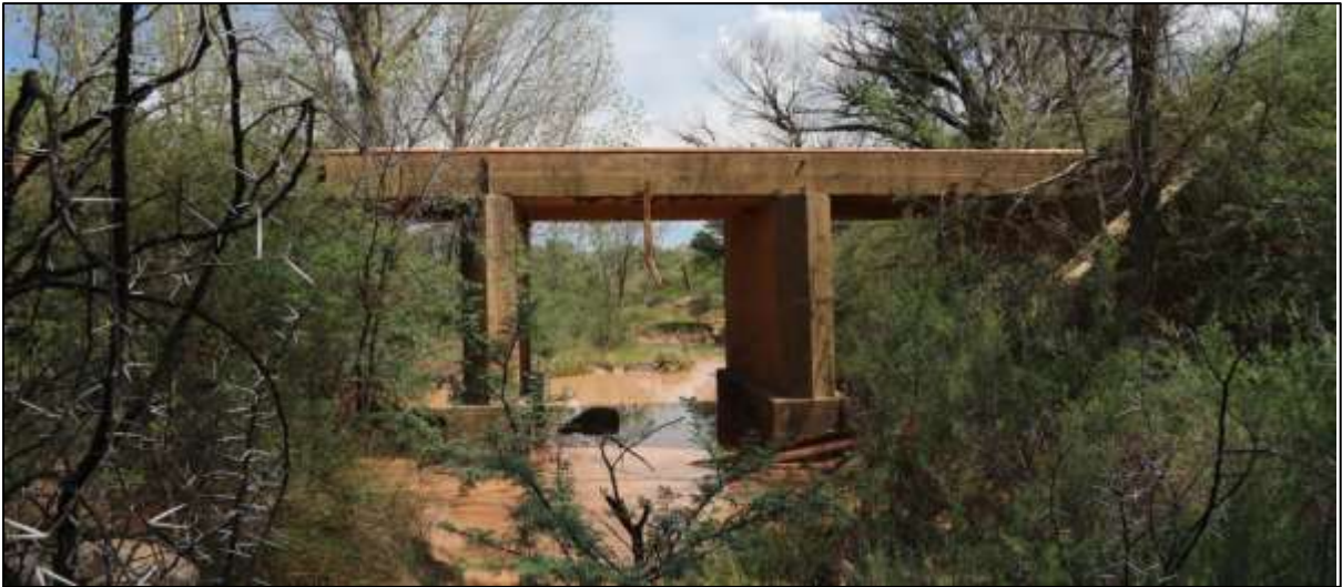
View of the gravel road and bridge over the Sandspruit. This will clearly have some impact in terms of flooding and scouring.
