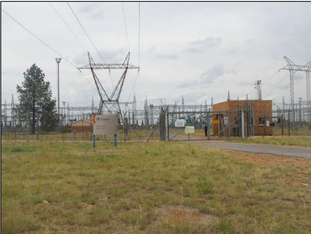
Figure 7: View of the Watershed Main Transmission Substation (MTS), which can be found within the corridor
