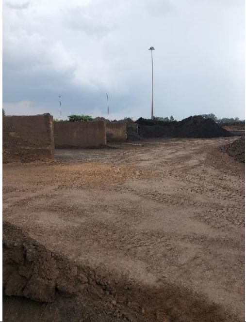
View of Briquetting Plant bunkers
